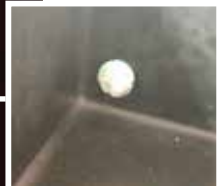
Underdrain outlet in the planter
